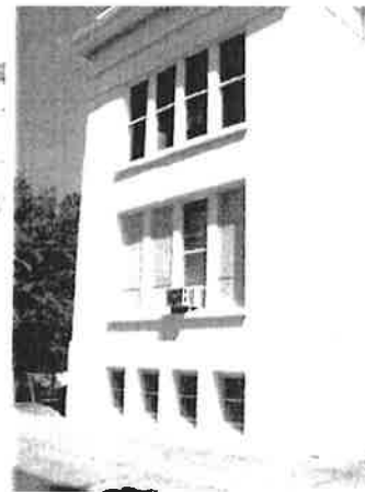
Photo 5.3: Window mounted air-conditioning units on the front side of the building.
